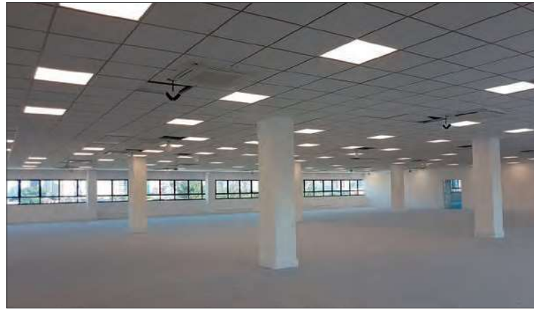
Efficient control of 1600 lighting ballasts is provided.
