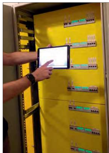
Cabinet operation being controlled by tablet interface.
